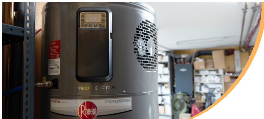
Heat pump water heater installed at the home of ENS customer.
