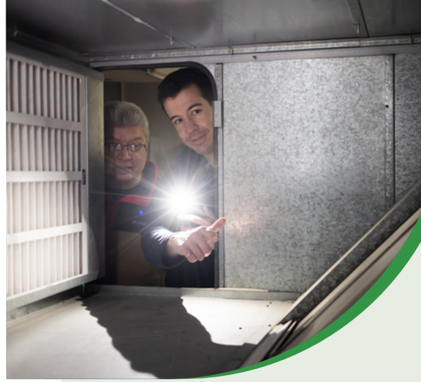
Quentin Doucette, Director of Public Works for Potlotek First Nation and Efficiency Nova Scotia Energy Manager Matthew Paul inspecting air vents.
